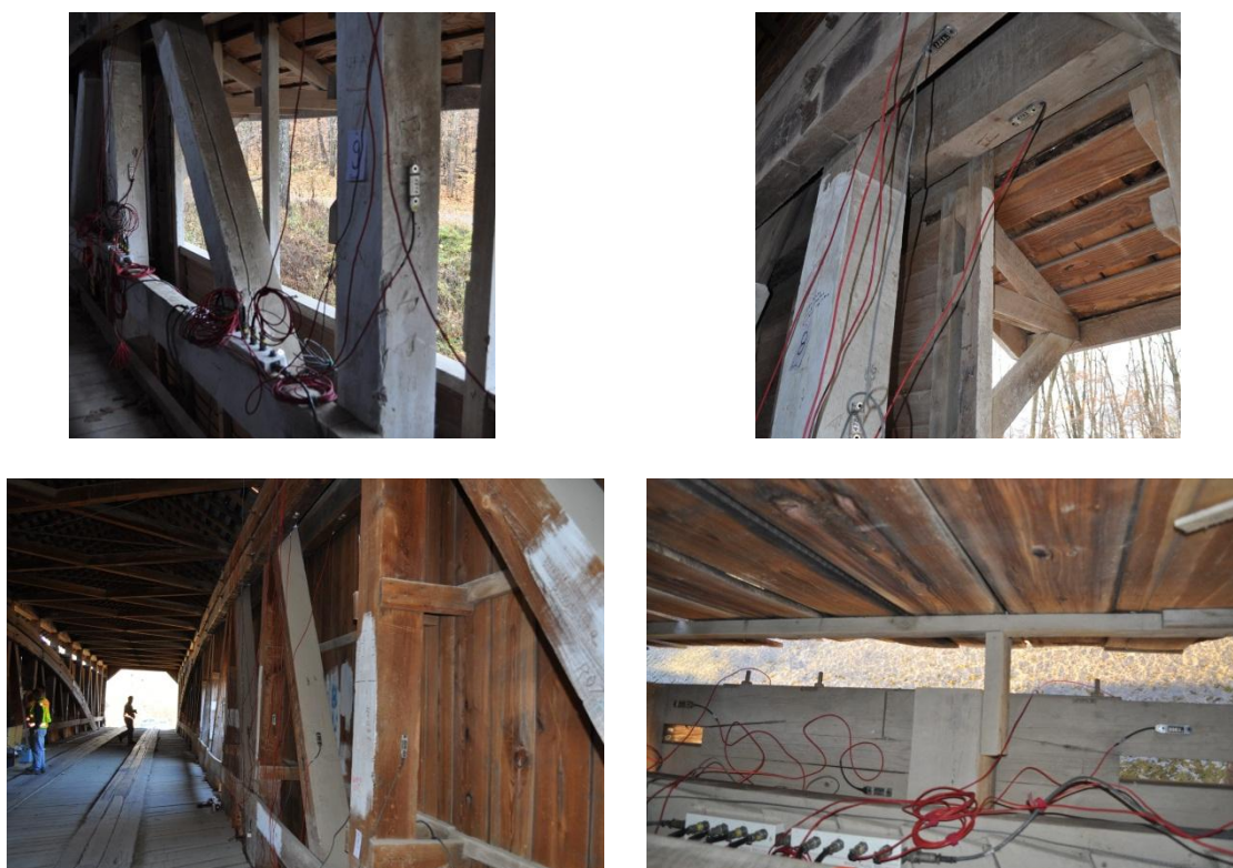
Figure 3.25: Typical strain transducer testing set up (top left is of multiple verticals, top right is underside of double concentric arch and vertical, bottom left is of multiple verticals and diagonals and bottom right of a splice joint in the bottom chord)
