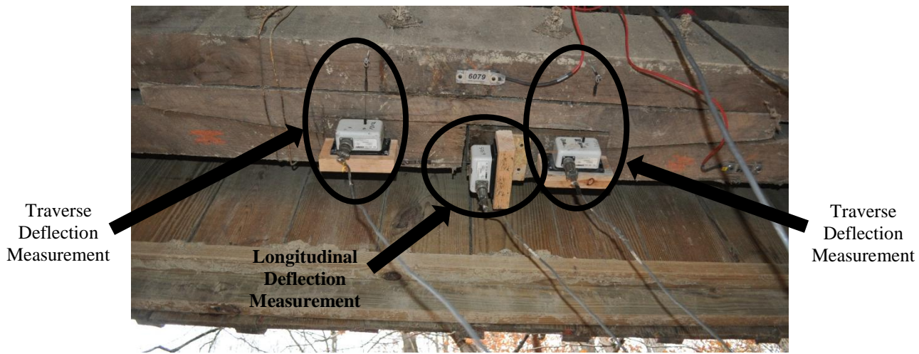
a. Photograph of the bottom face of the bottom chord displacement measurements
