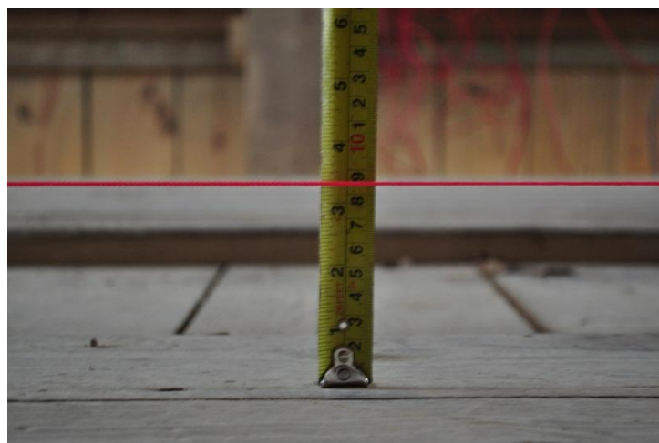
c. Pre-existing sag in the overall bridge with measurement at mid-span
