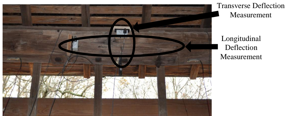
a. Photograph of the elevation view of the top chord displacement measurements
