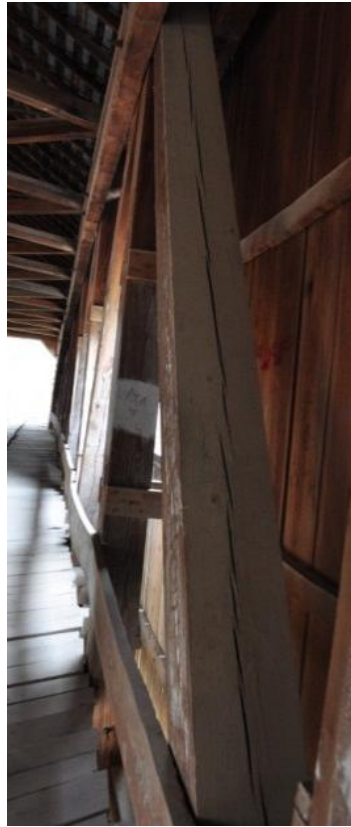
c. Length and depth of checks within timber members
