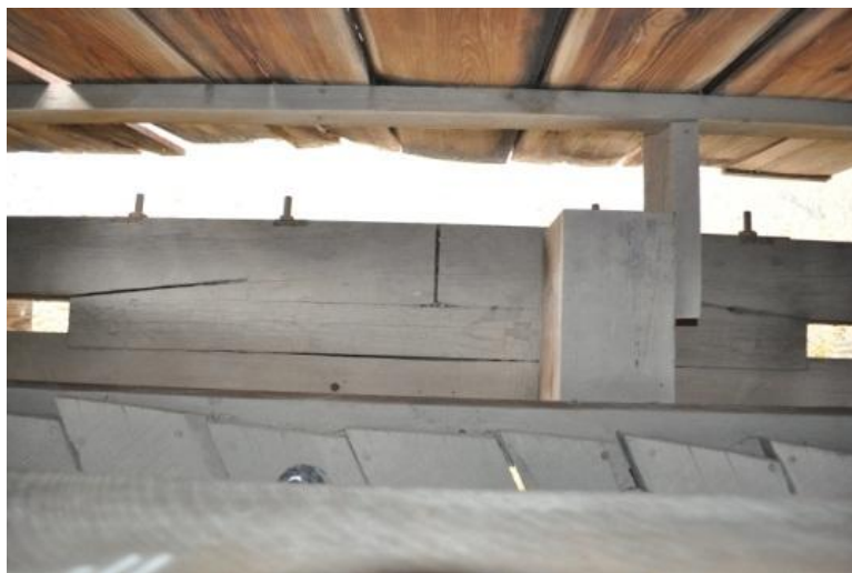
a. Gaps within the interface between the bottom chords and splice joint
